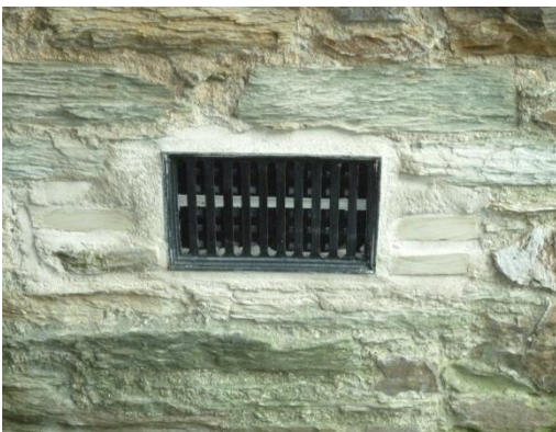
Double Anti-Flood Airbrick, installed behind existing grill to listed property
