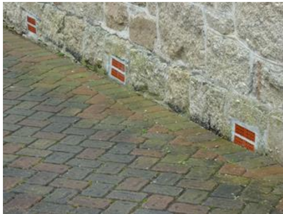
Double Anti-Flood Airbrick in situ
