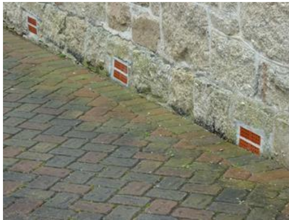
Double Anti-Flood Airbrick in situ
